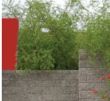
This wall shows a layering of CMU and stucco finishes to provide contrast and identity.
